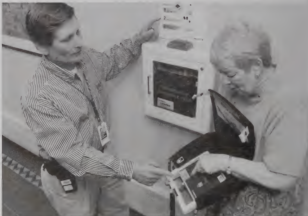
Fredrick Manuel and Jerry Taylor demonstrate the easy-to-understand instructions of one of the new automatic external defibrillators stationed outside of the second floor cafeteria. Thirty-five of the plexiglass AED stations have been placed throughout the Clinical Center. NIH CPR training is required to use the device.
