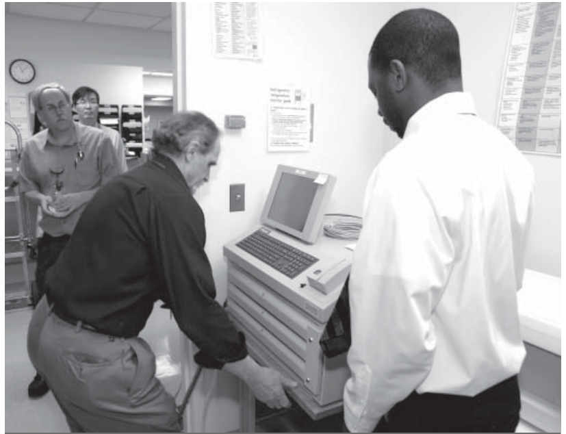
The first cabinet was installed in Outpatient Clinic 3 on April 6. Pharmacist Thomas Dorworth (middle) and Omnicell technician Ryan Wiggins (right) move the machine into its new space while pharmacists Barry Goldspiel (left) and Jae Kim look on.
