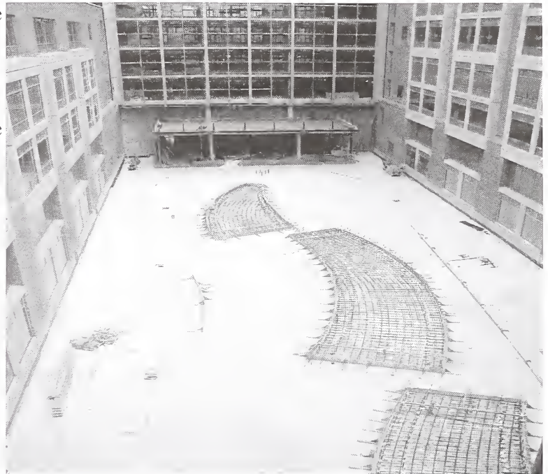
One of the two inner courtyards to the CRC now is cement. Dirt, trees, bushes, and a fountain will create a serene and private environment for patients and visitors.
