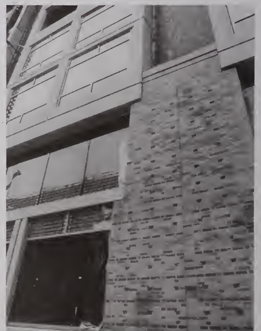
Ground was broken for the Clinical Research Center on Nov. 4, 1997. Projected completion is March 2004.
