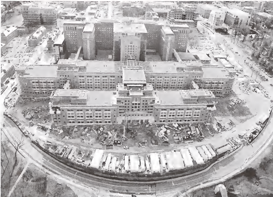
Aerial photo taken in early January of the Mark O. Hatfield Clinical Research Center with the building exterior virtually complete.
