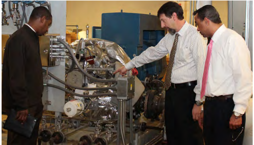
Donald Edwards (left), chief of the NIH Clinical Center's Facilities Branch, Greg Leifer (center), with the Energy Management Branch, and Michael McClain (right), the facility manager for Building 10, gather at the Clinical Center's new steam turbine recently installed in the basement of the hospital. The new equipment, which provides heat to the hospital by converting steam to mechanical energy, will reduce power consumption by using it more efficiently, thereby saving costs. This modern and easier-to-operate equipment replaces the old turbine installed during the building's construction in the 1950s. The new turbine will provide an estimated 2.4 million kilowatt hours of electricity, equivalent to enough electricity to power 200 average-size homes per year. This upgrade is anticipated to save approximately $200,000 per year.
